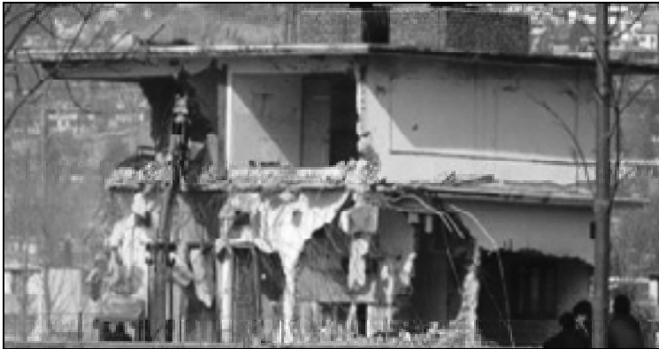
DEMOLITION ZONE: Cops stand guard as former al-Qaida supremo Osama bin Laden's safehouse in Abbottabad is demolished.
